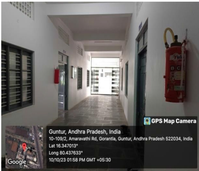
Fire Extinguisher at Labs
