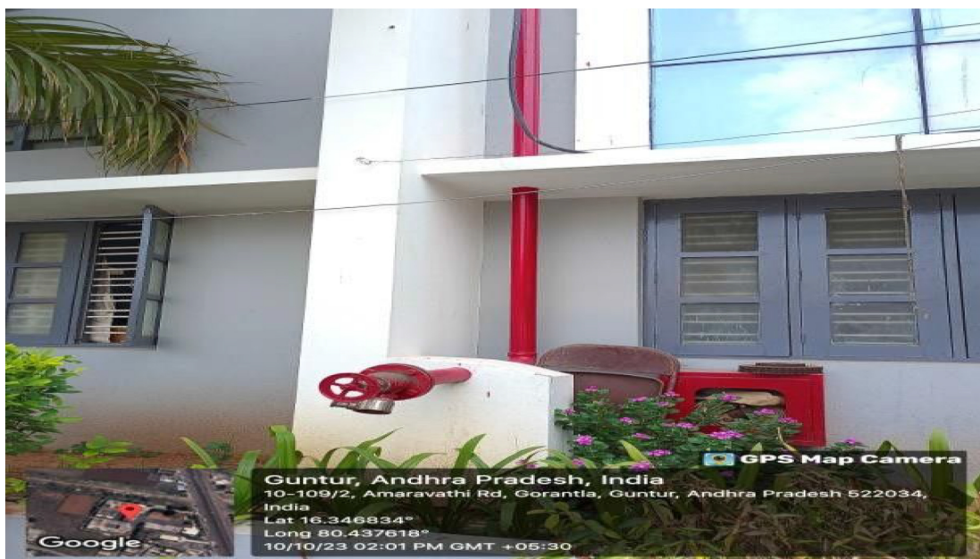
Fire Hydrant Valve
